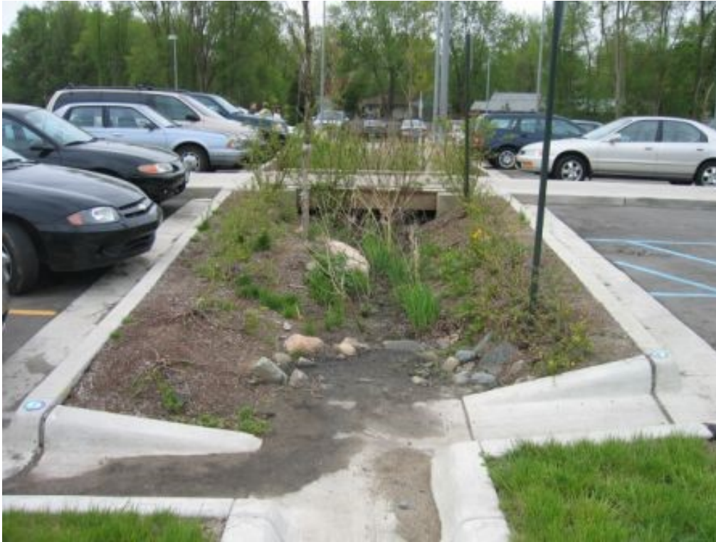
Figure 3: Bioretention Area that needs maintenance to address dead and unhealthy vegetation within the main treatment area.
