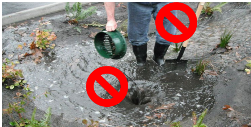
Figure 4: Bioretention Area that needs maintenance to address a clogged outlet structure.
